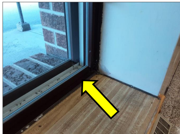
Asbestos-containing hard brown caulking.
