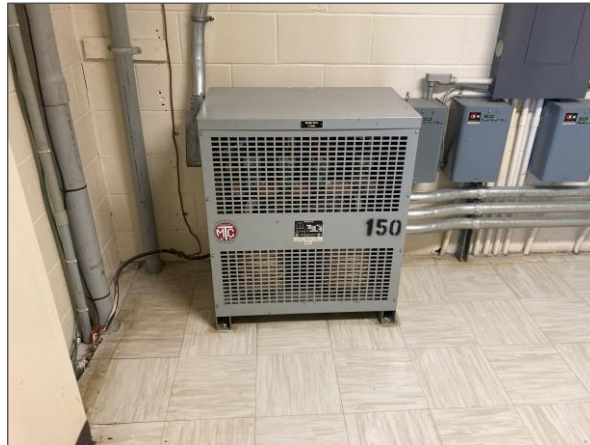
Non-PCB dry type transformer.
