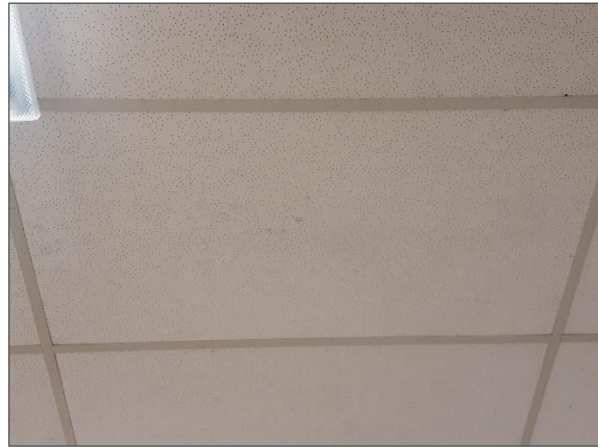
Non-asbestos lay-in ceiling tiles with small and medium pinholes.
