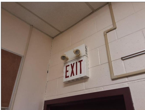
Lead-containing batteries in emergency lighting.
